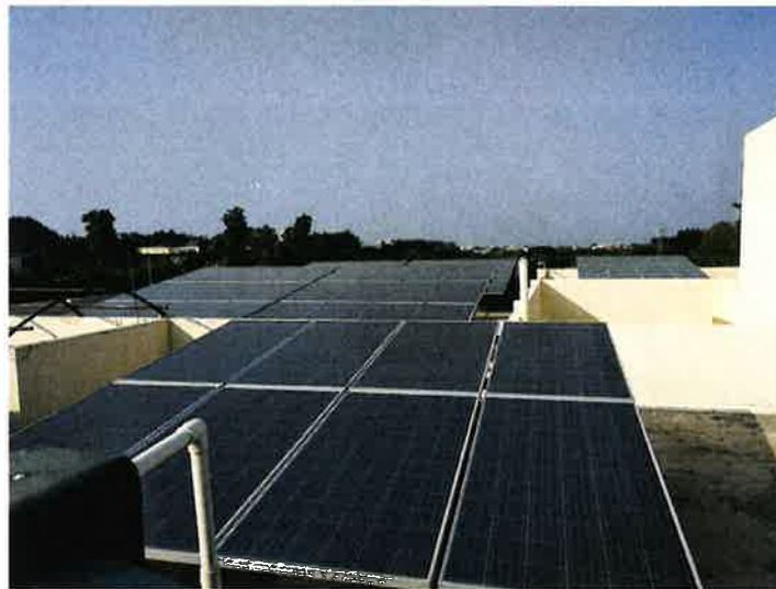
Roof Top Solar Plant – 30 kWp
